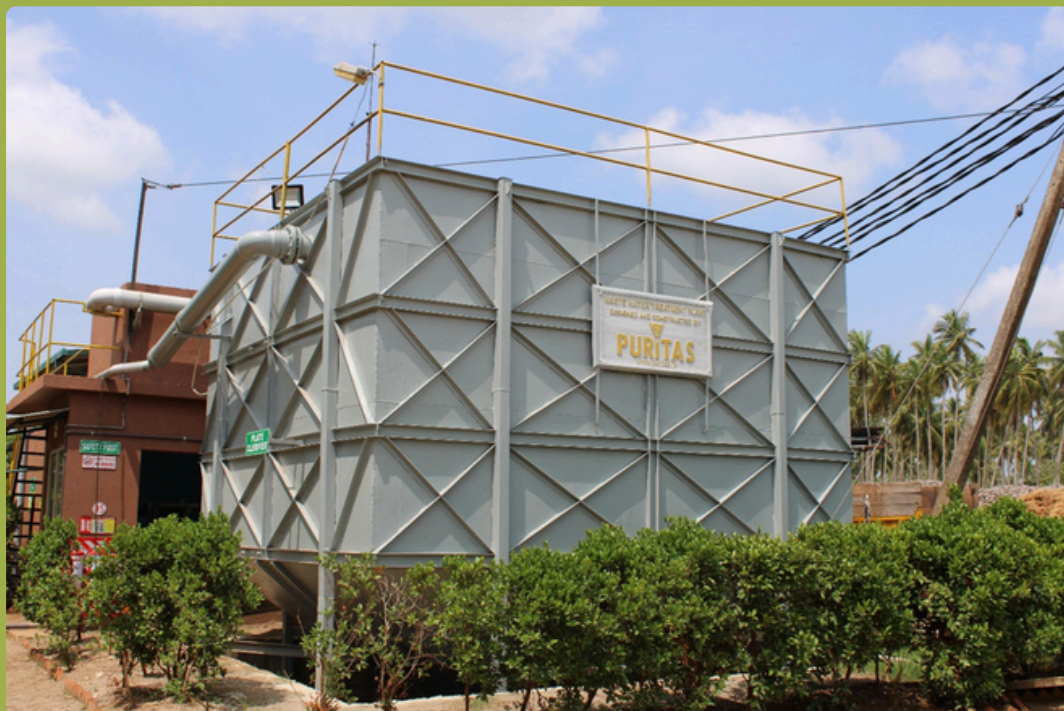
Our wastewater treatment plant
